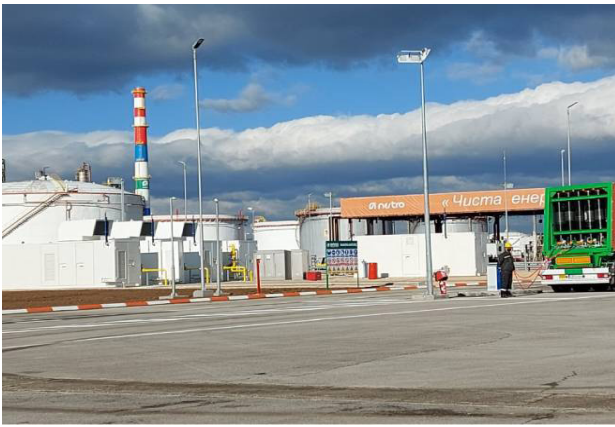
Figure 3. The compressor gas station in "Oil Refinery Brod a.d." Brod
