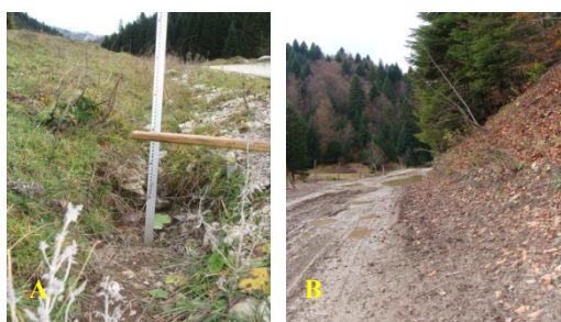
Figure 2. A- The cleansing needed, B- The digging of ditches needed (photo org. Halimić, 2012)
