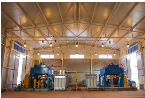
Figure 1. The compressor plant in the company "Prvo gasno društvo" Zvornik
